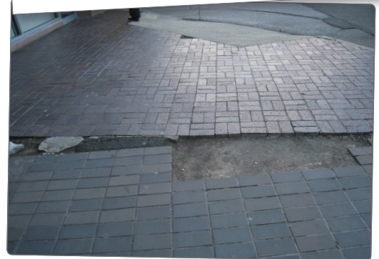
Sidewalks are sometimes poorly maintained outside of the pedestrian core (Broad Street)
